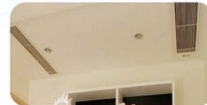
Front air flow, back air intake
